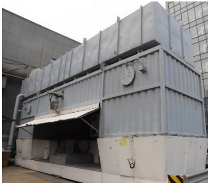
Waste gas treatment facilities of painting workshop - Regenerative Thermal Oxidizer (referred to as 'RTO'). The waste gas collection rate of fully enclosed painting line is 95%, and the RTO treatment rate is 90%.
