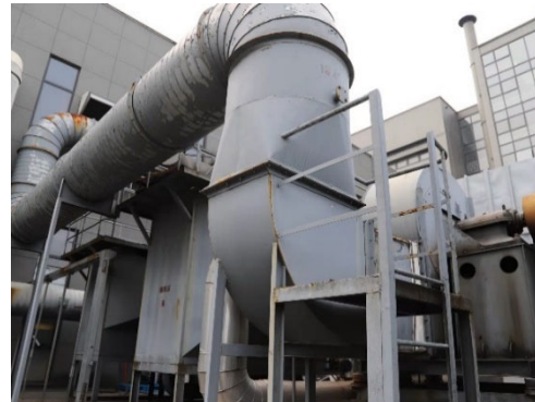
Waste gas treatment facilities of painting workshop - Regenerative Catalytic Oxidizer (referred to as 'RCO'). The waste gas collection rate of the fully enclosed painting line is 95%, and the RCO treatment rate is 90%.
